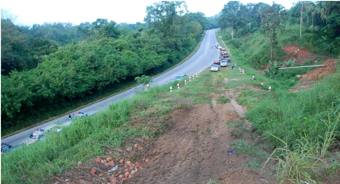
Figure 3-16: Ramp Condition after Crash
